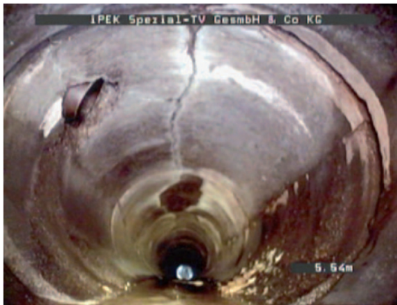
old and damaged sewer
